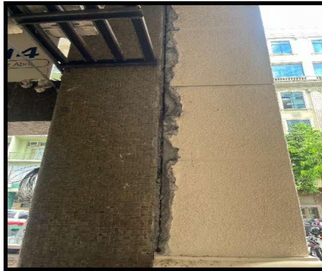
Figure 4. Visual inspection of the Aminco Amaya building, where structural damage was identified
